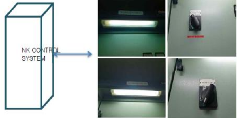
NO1, 2 Fire Bilge GS Pump
